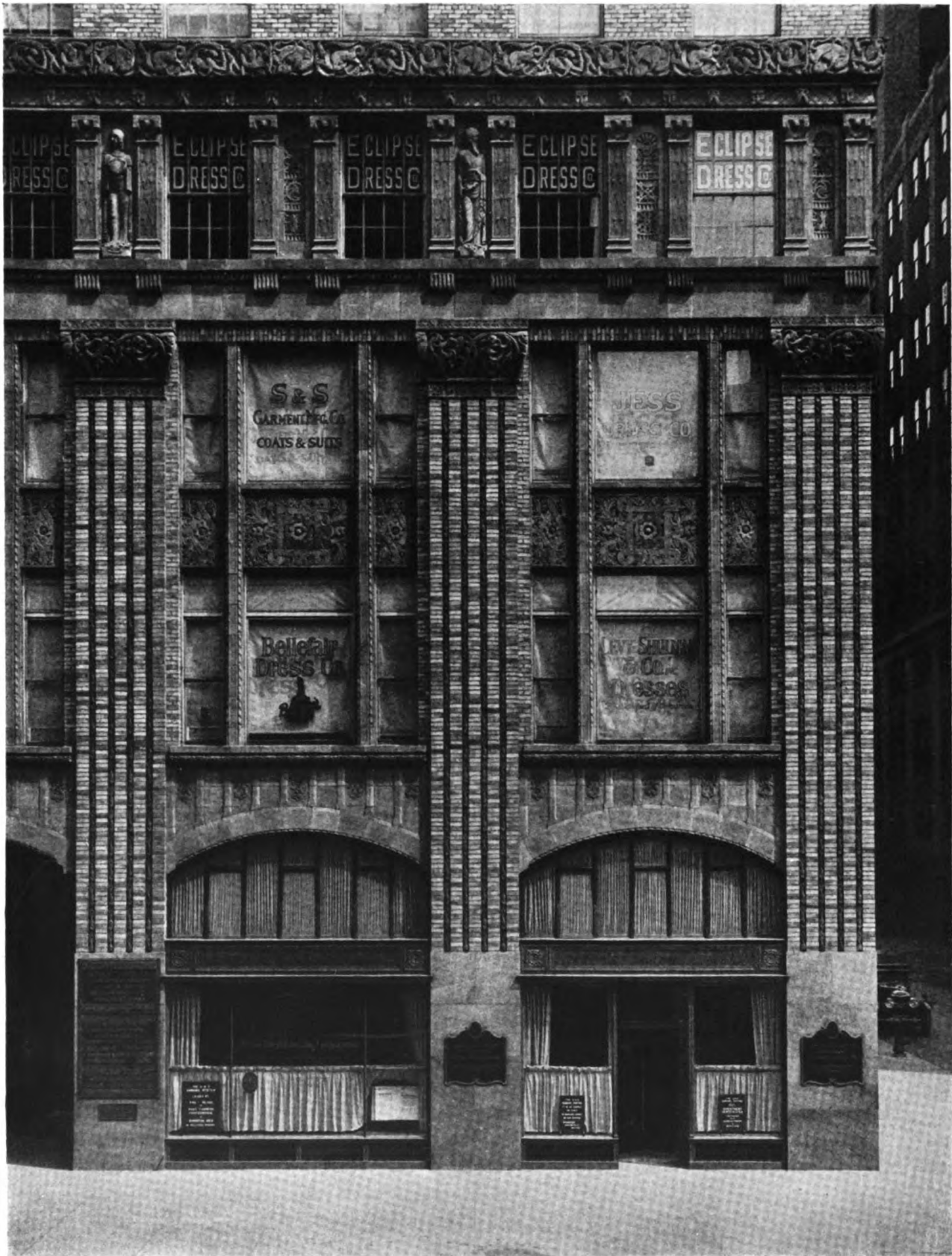
DETAIL OF BRICKWORK, LOWER STORIES ARSENAL BUILDING, SEVENTH AVENUE, NEW YORK BUCHMAN & KAHN, ARCHITECTS
